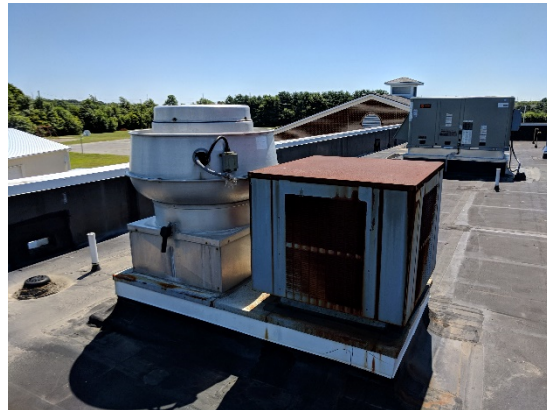
Photograph #2 – Kitchen Ventilation Unit
