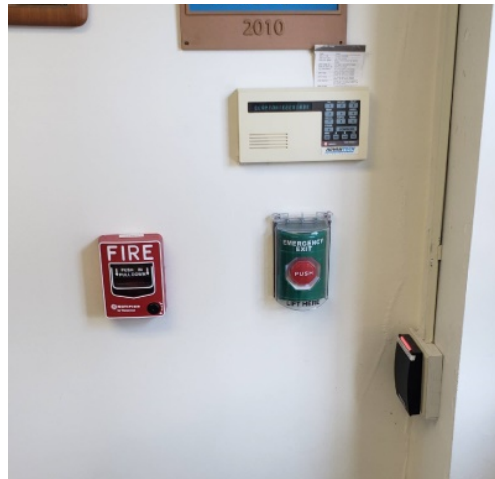
Photo #11 Fire Alarm Pull Station, Card Reader, and Security Keypad
