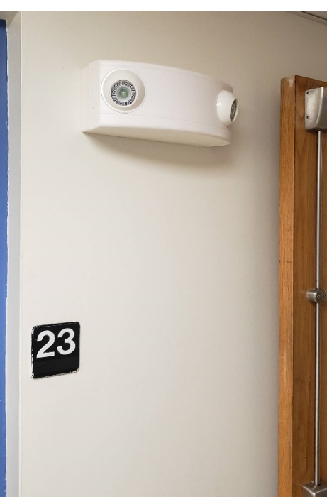
Photo #6 Typical Wall Mounted Emergency Light
