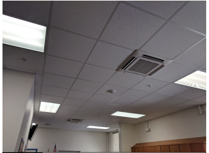
Photo #2 Ceiling Cassettes-Front Office
