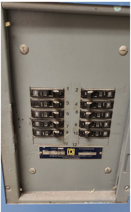
Photo #4 Panelboard LPB
