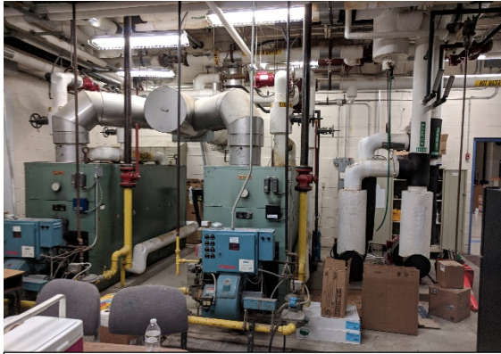
Photograph #1 – Boilers in Mechanical Room
