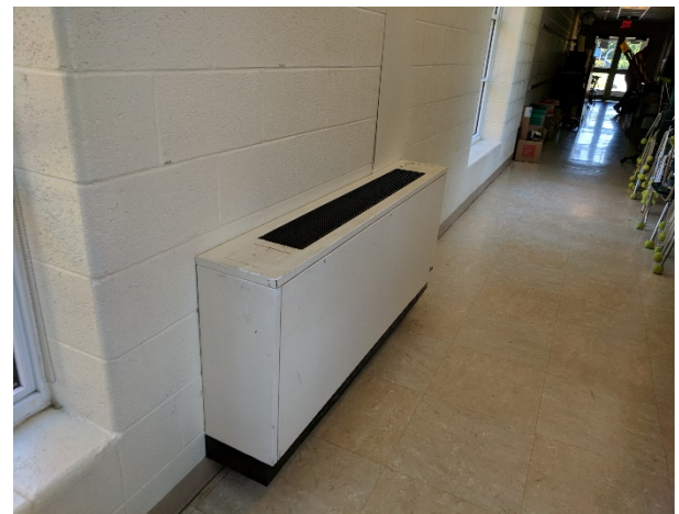
Photo #15 Typical Fan Coil Unit
