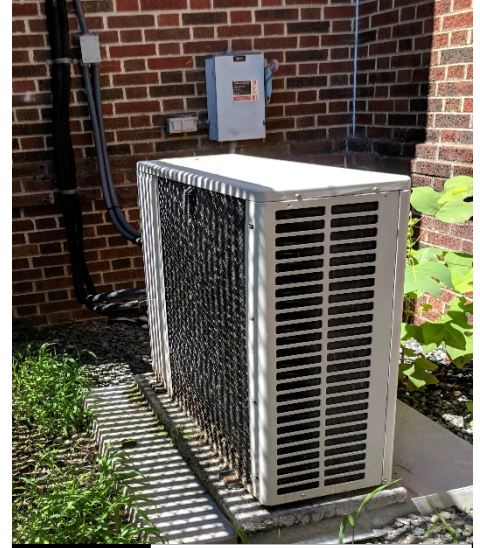
Photo #9 Exterior Disconnect on Wall
