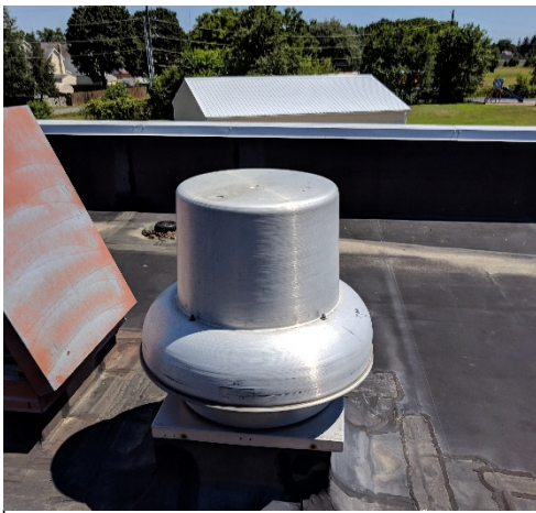
Photograph #3 – Typical Exhaust Fan
