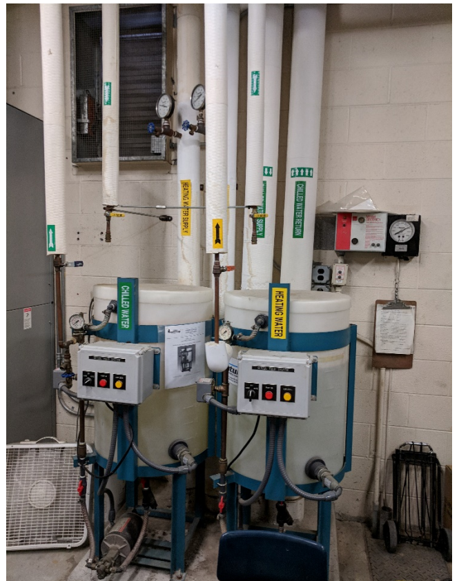
Photo #4 Chilled and Heating Water Glycol Feeders in Mechanical Room
