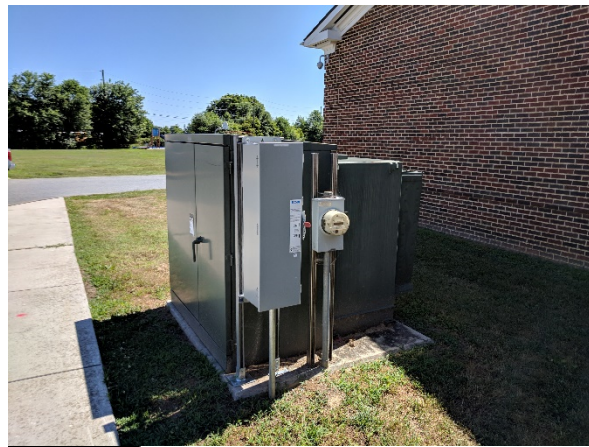
Photo #16 Transformer, Meter, and Disconnect for Fire Pump
