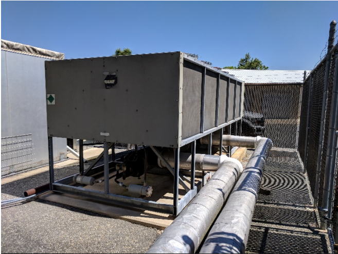
Photo #1 Air Cooled Chiller in Mechanical Yard
