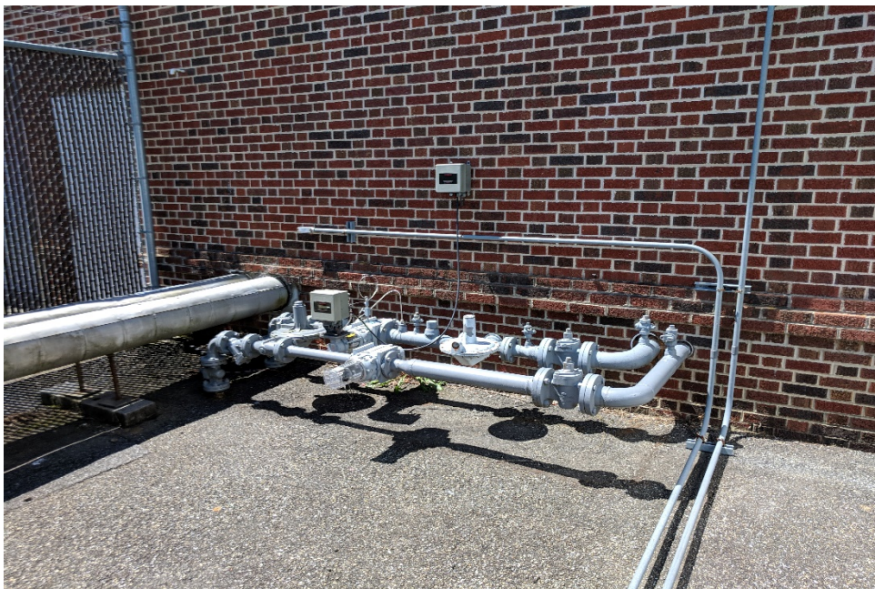
Photo #7 Gas Meter
