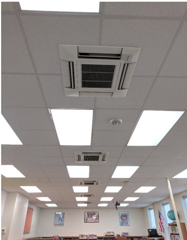
Photo #3 Ceiling Cassettes-Library
