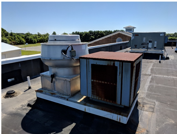
Photo #10 Kitchen Ventilation System
