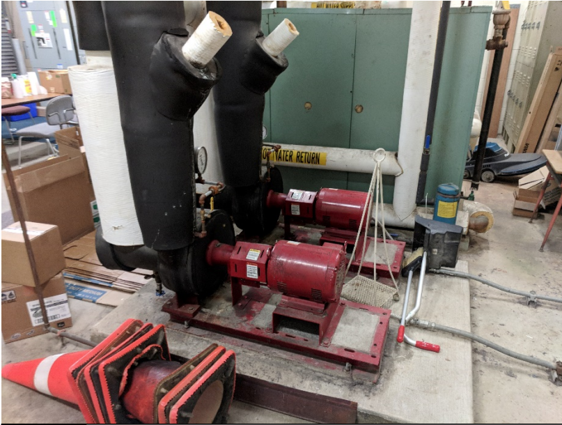
Photo #5 Chilled water Pumps in Mechanical Room
