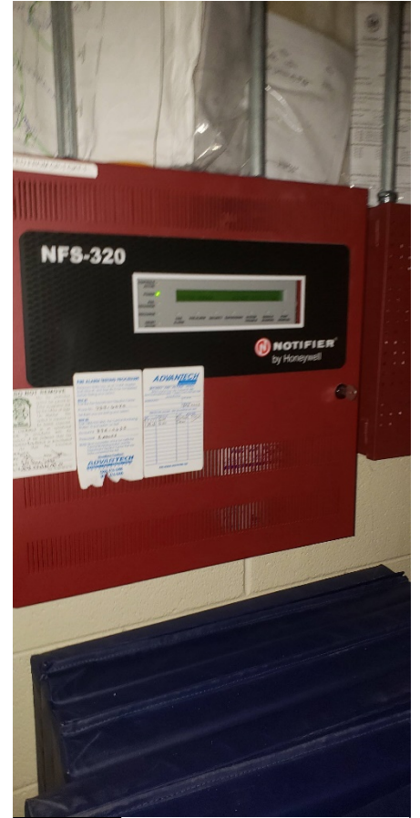
Photo #3 Fire Alarm Control Panel
