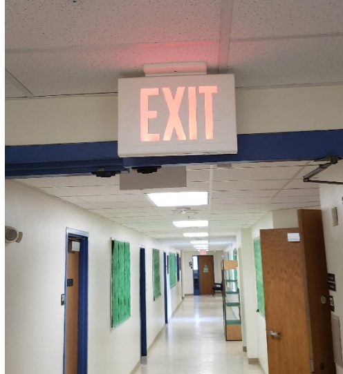
Photo #8 Typical Exit Sign & Recessed Lighting In Corridors
