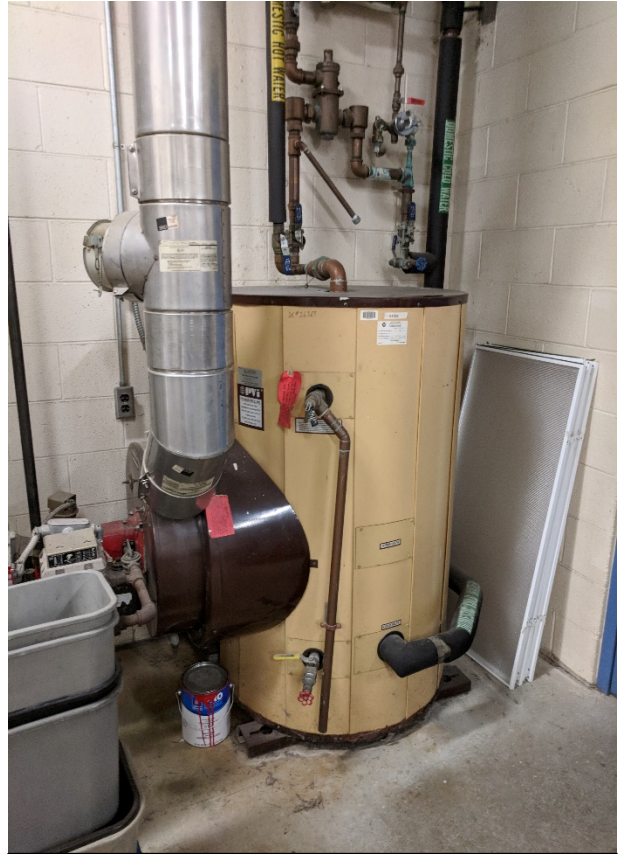
Photo #6 Domestic Hot water Heater in Mechanical Room
