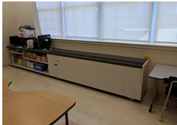
Photograph #4 – Typical Classroom Unit Ventilator
