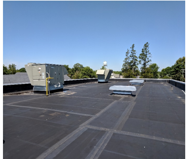
Photo #13 RTUs serving Cafeteria, Gym, and Auditorium
