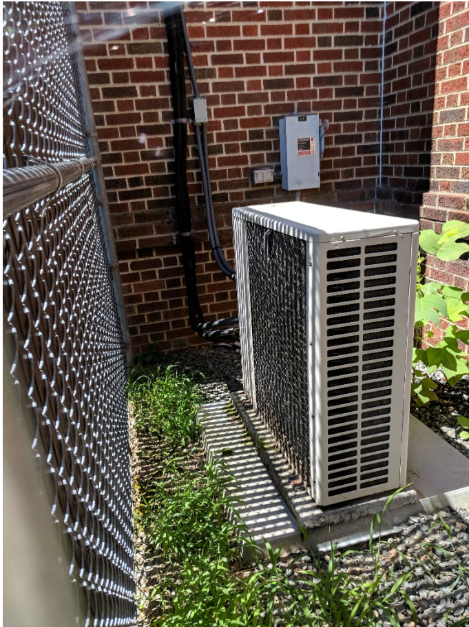
Photo #8 Ground Mounted Split DX Condensing Unit
