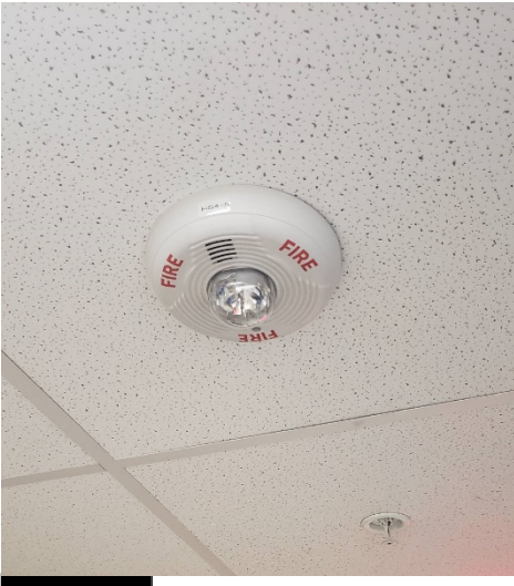
Photo #7 Typical Ceiling Mounted Fire Alarm Device
