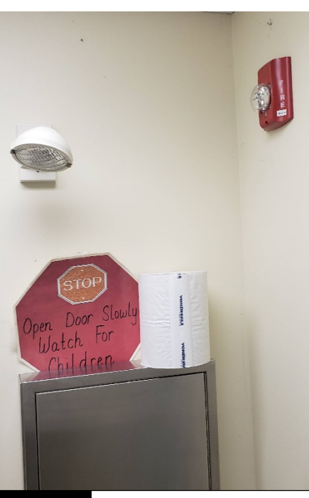
Photo #5 Wall Mounted FA device in typical Bathroom
