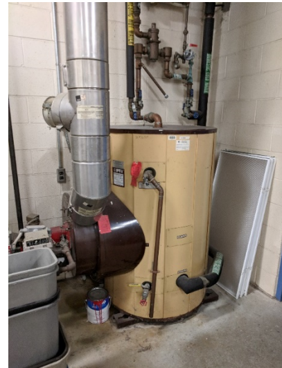
Photograph #5 – Water Heater
