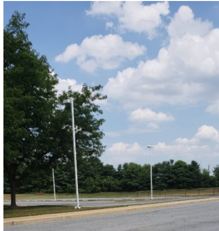
Photo #14 Typical Parking Lot Pole Lights
