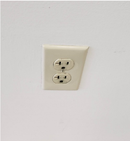
Photo #10 Typical Receptacle
