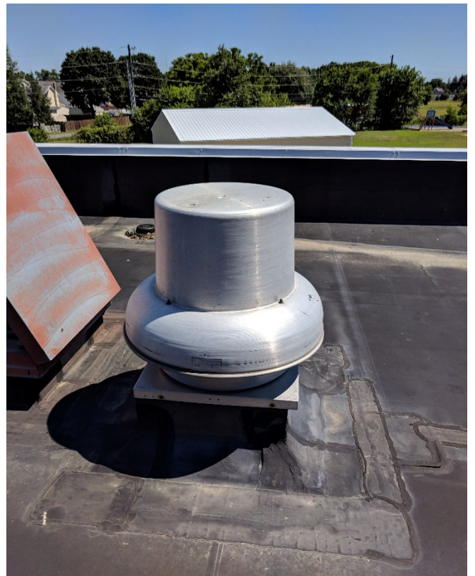
Photo #11 Typical Roof Mounted Exhaust Fan
