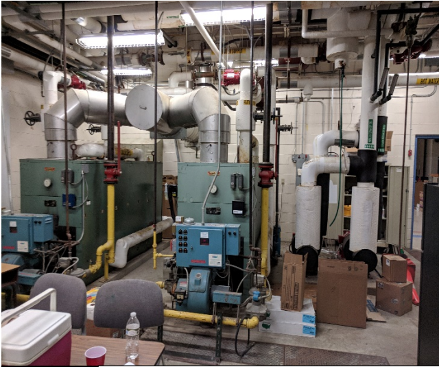
Photo # 12 Boilers in Mechanical Room
