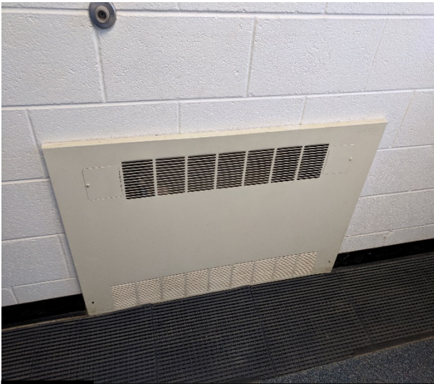
Photo #14 Typical Cabinet Unit Heater
